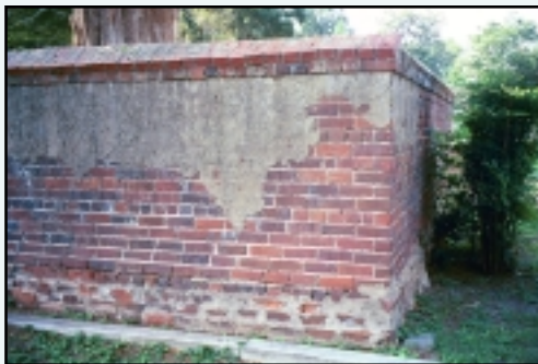
This wall has been inappropriately repointed with Portland cement that extends beyond the original mortar joints.
