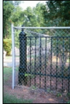
Chain link fencing is a modern intrusion into the historic cemetery.
